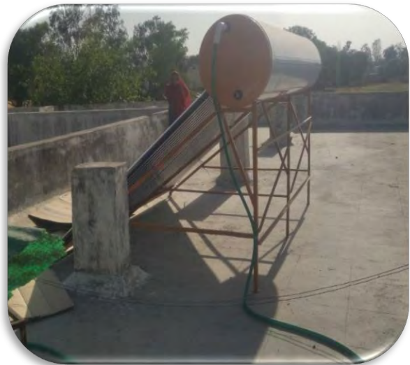
Solar Water Heaters
