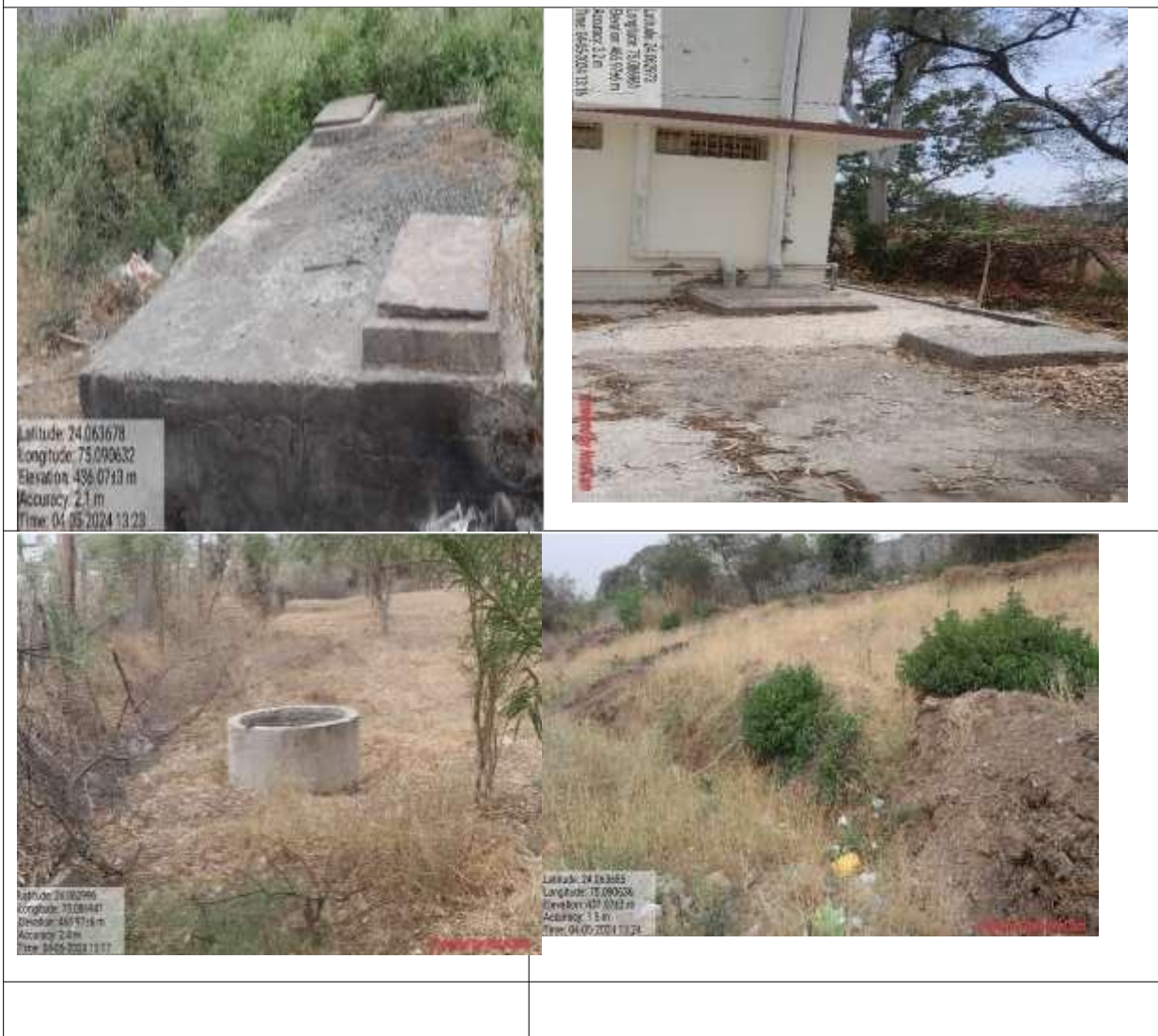
Septic tank for waste water of colleg
