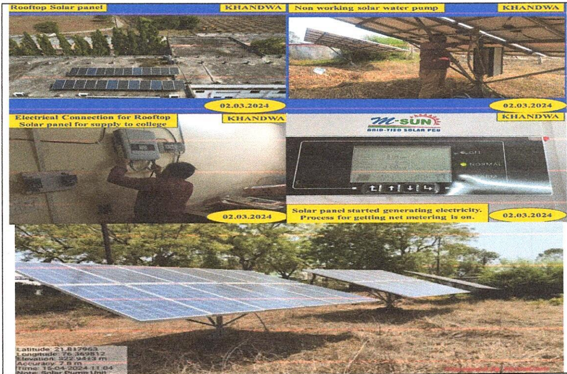
Electricity generation from solar units
